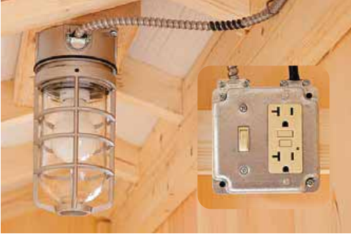
Electric Package - Switch / Outlet / Lights Extension Cord Hookup
