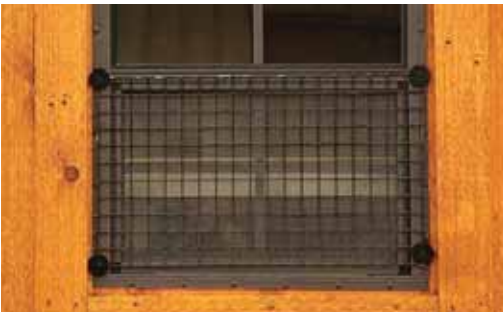
Wire over window
